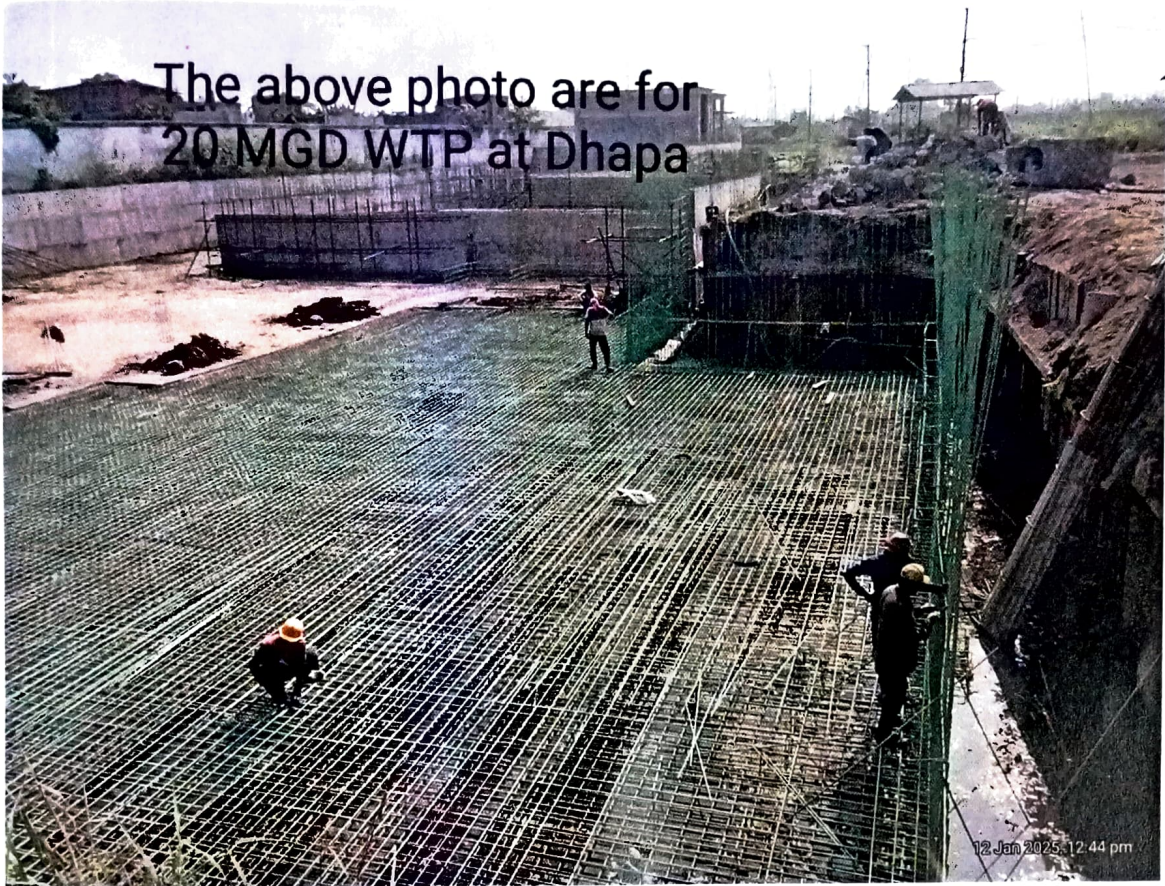
The above photo are for 20 MGD WTP at Dhapa
