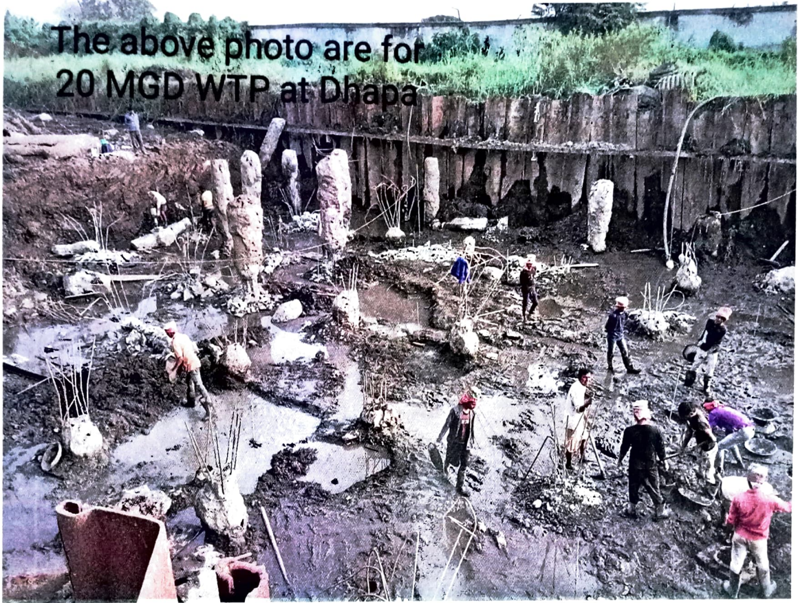
The above photo are for 20 MGD WTP at Dhapa
